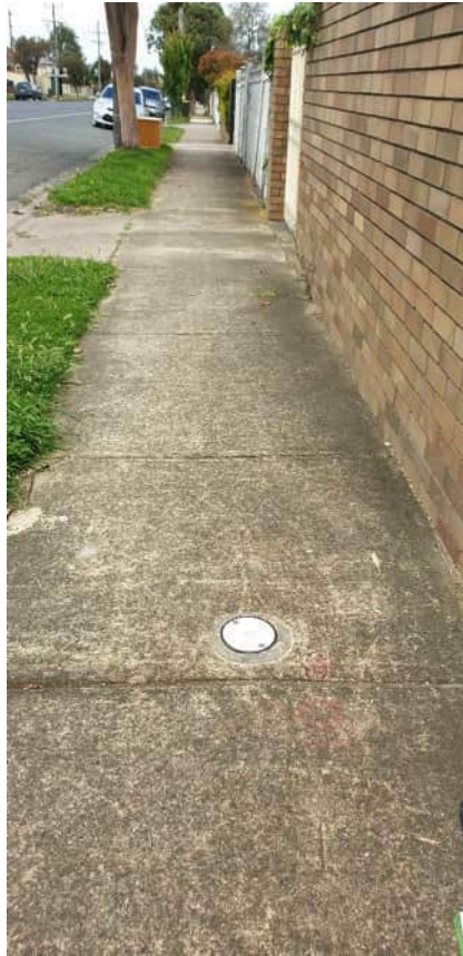
Photograph C.21: N-LFG-01 installed location (Newtown closed landfill)
