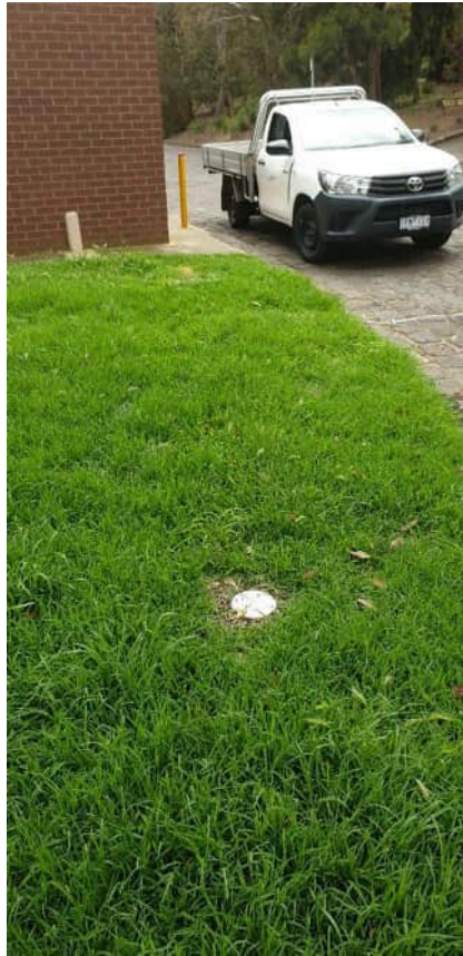
Photograph C.15: L-LFG-05 installed location (Leech-Wood Gardens)
