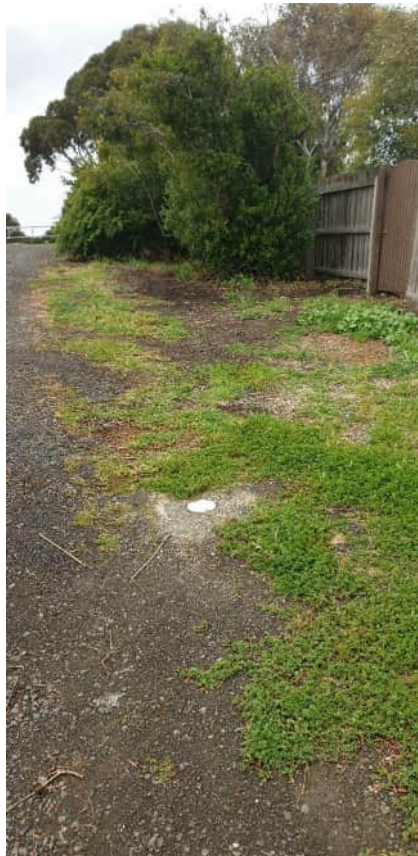
Photograph C.2: W-LFG-03 installed location (Windmill Reserve)
