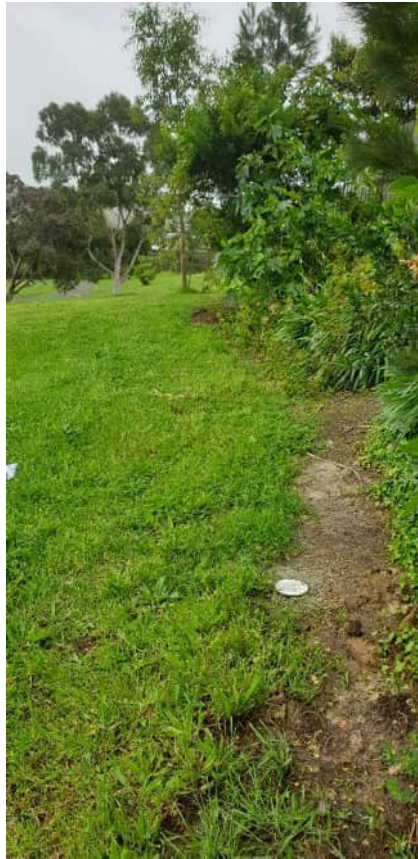
Photograph C.3: R-LFG-01 installed location (Rotary Centennial Park)
