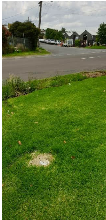
Photograph C.27: N-LFG-07 installed location (Newtown closed landfill)
