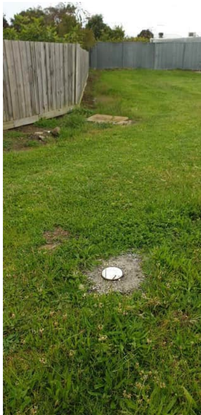
Photograph C.6: R-LFG-04 installed location (Rotary Centennial Park)
