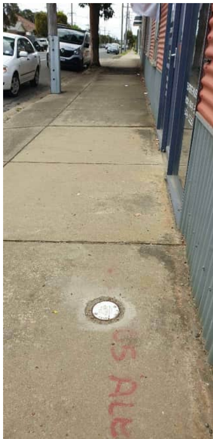
Photograph C.20: M-LFG-05 installed location (Marnockvale closed landfill)
