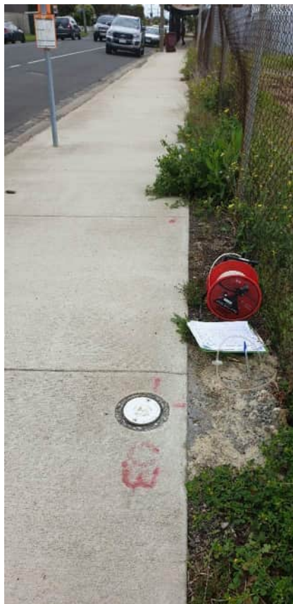
Photograph C.18: M-LFG-03 installed location (Marnockvale closed landfill)
