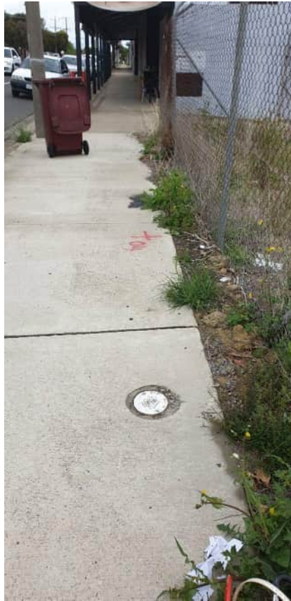
Photograph C.19: M-LFG-04 installed location (Marnockvale closed landfill)
