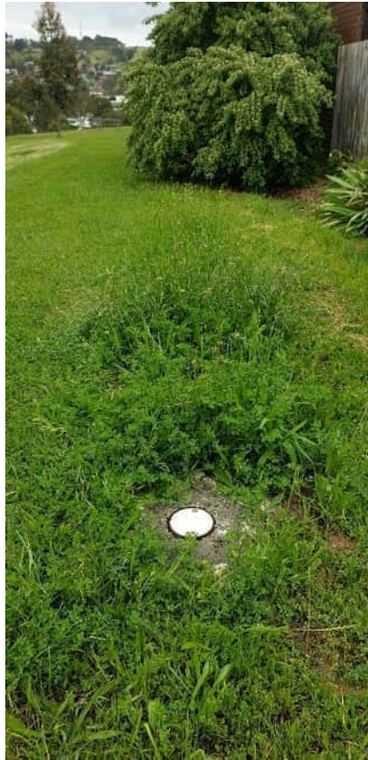
Photograph C.5: R-LFG-03 installed location (Rotary Centennial Park)
