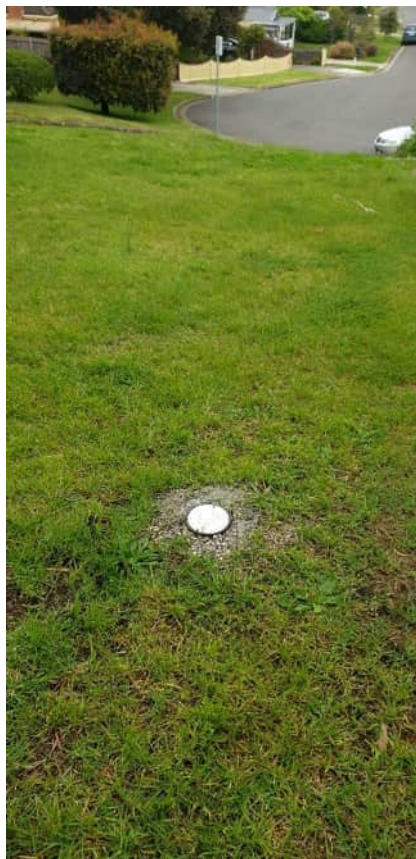
Photograph C.12: L-LFG-02 installed location (Leech-Wood Gardens)
