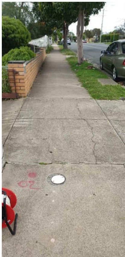
Photograph C.22: N-LFG-02 installed location (Newtown closed landfill)
