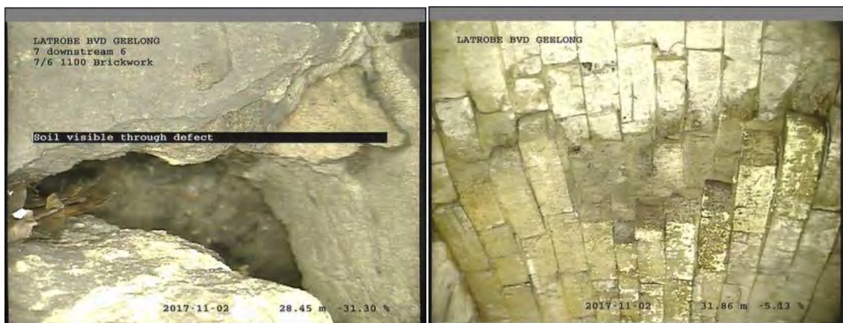
Figure 3.5 CCTV photographs showing defects on the Latrobe Boulevard alignment
