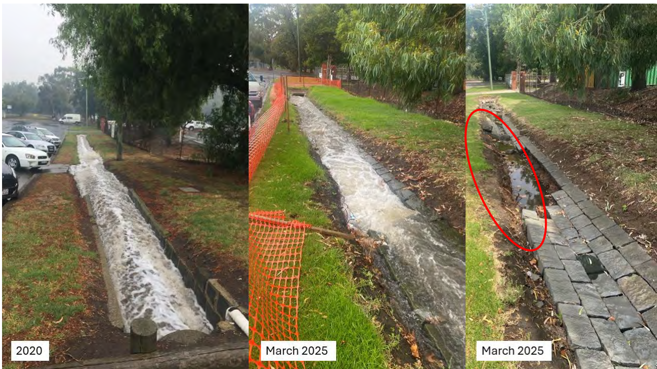
Figure 3.8 Blue stone open drain on Bellerine St in 2020 and further eroding after a storm in March 2025
