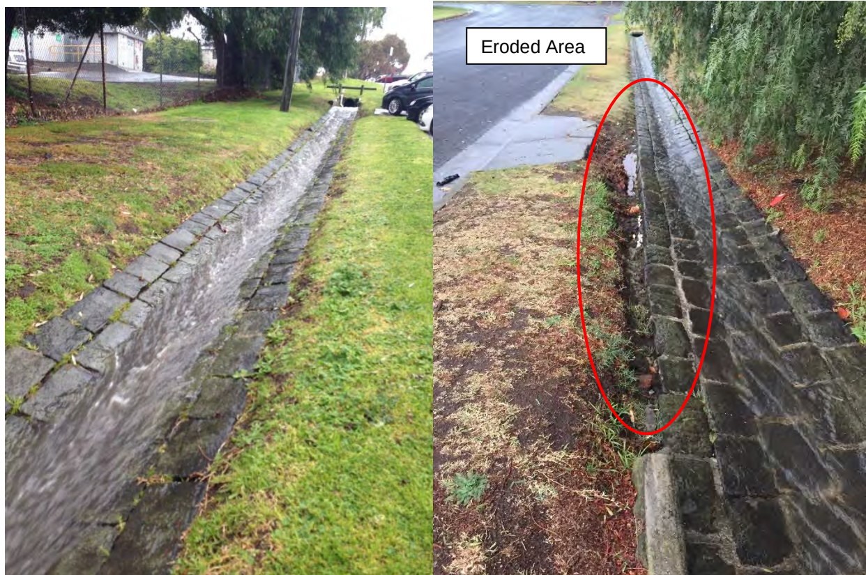
Figure 3.7 Blue stone open drains on Bellerine St 2018 (during a storm event), Right: outflanked area that is becoming undermined
